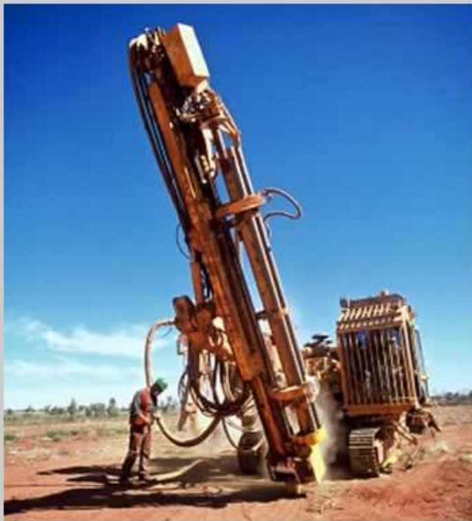
The rig will also be used to drill the Namwele deposit and Muze portion of the Rukwa Coalfield Project in South Western Tanzania.
